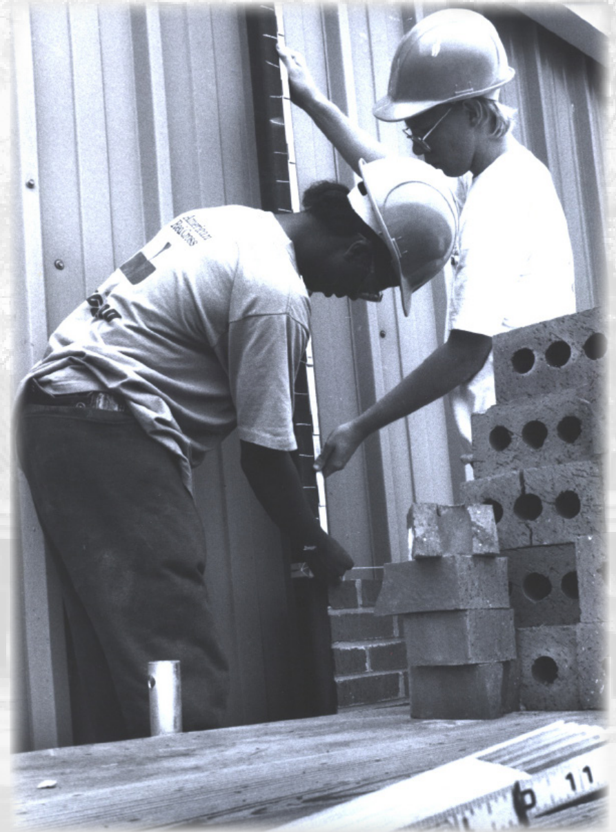
Instructor John Nail's Construction Trades students practice their masonry skills while dressing up a metal structure on the northeast side of the El Reno campus.
